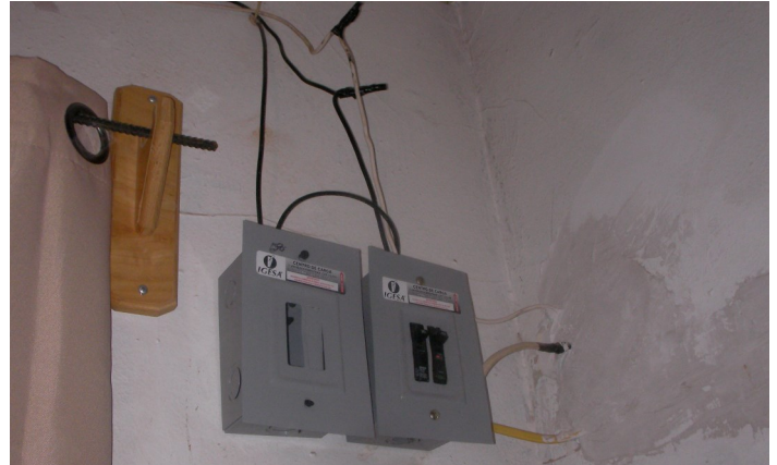
Electrical upgrades are badly needed at two sites in Juarez.
